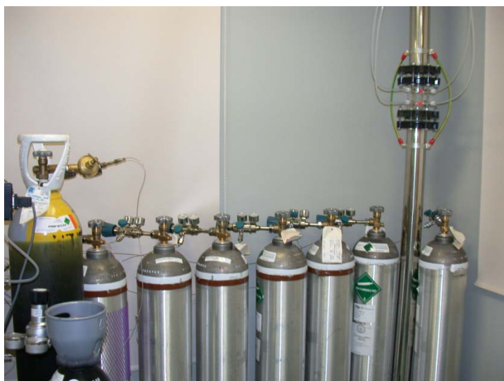
Fig. 4 : Sample air inlet for trace gas analysers with manifold in the laboratory of the 3 rd floor of the Izaña station building. The picture also shows the set of laboratory standards for N 2 O (see 3.6.2).
